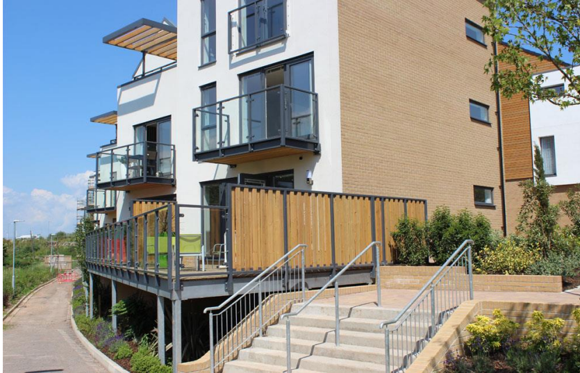
Typical external domestic welded / fabricated steelwork
